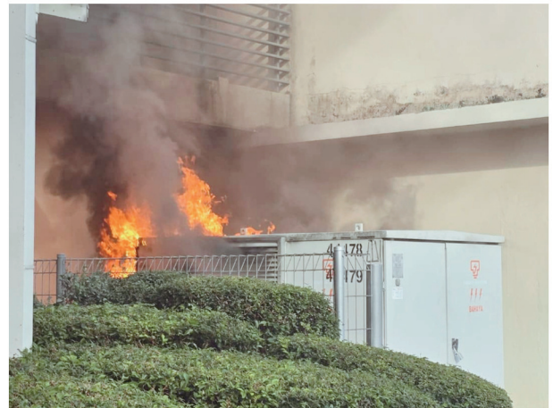
Ecumenical Centre Substation Engulfed In Flames
